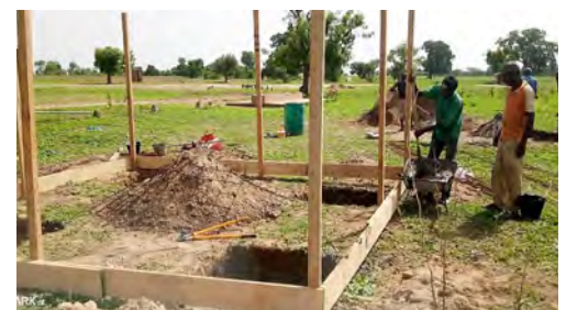
Excavating and framing the solar pump house. This structure will hold the solar panels and above ground water reservoir.
