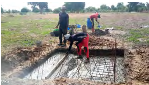
Masons pour the foundation of one of the watering basins. There are a total of five in each garden.
