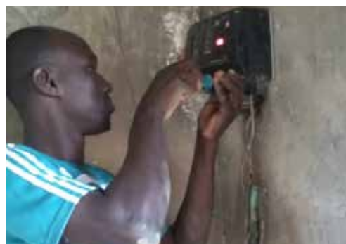
Maintenance Technician Hamath repairing a solar pump controller. This new staff position supports garden participants in long-term care of garden infrastructure.
