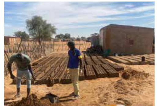
It is exciting to see the construction progress! Bricks are made on site, and soon the structure will start to rise up.
