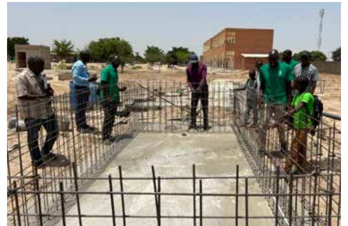
Construction is nearly complete on our first-ever school garden at Keur Soce High School, which will be the first high school in all of Senegal with an integrated aquaculture training program.
